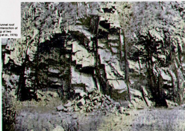
Figure 4.28 Rock falls caused by closely spaced multiple joint sets, with one set daylighted, Golden Gate Canyon, Colorado.
