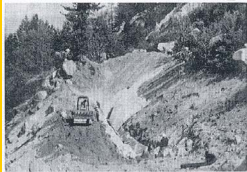
Figure 3.13 A bulldozer pulling a sheepfoot roller to compact the initial soil layers on a reinforced fill for a mountain road.
